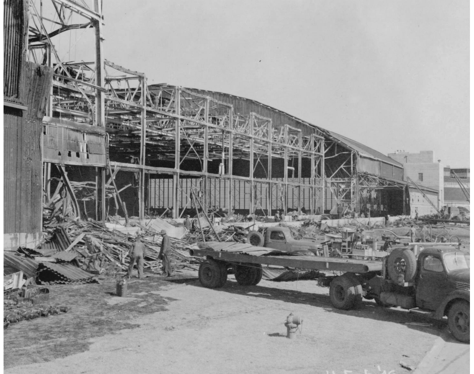
Construction after a fire on Tinker Air Force Base in 1946 (22596.12, Jacqueline D. Wright Collection, OHS).
