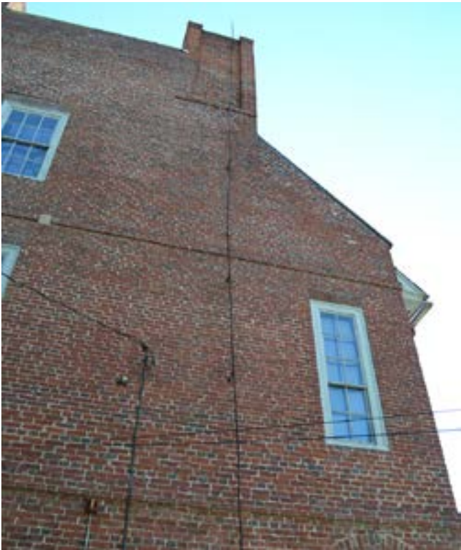
Figure 6. Lightning protection was installed on the Warner House in Portsmouth, New Hampshire, in 1767, purportedly under the personal inspection of Benjamin Franklin. An early system still survives on the building, consisting of a long forged-welded rod of wrought iron which extended up and above the chimney, comprising both the conductor and the air terminal. The conductor was joined to a separate, buried, iron ground rod by a forged hook and eye connector. Photo: Peter Michaud.
