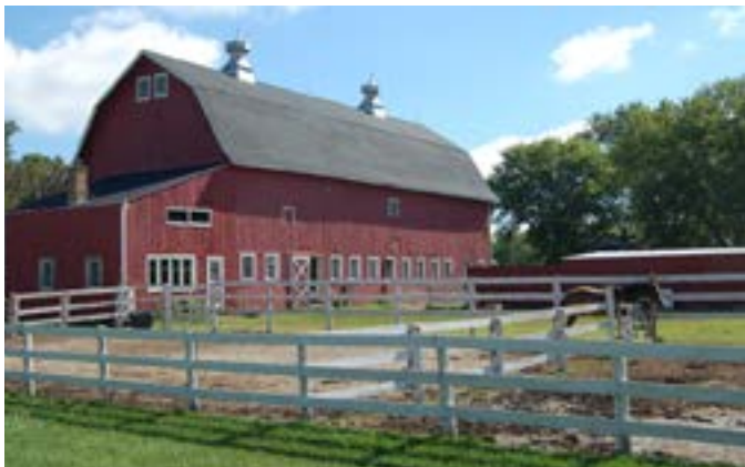
Figure 21. Small air terminals have been used in this more recent installation and have little visual impact. If a partially concealed system was desired, the cable and the mount for two of the air terminals could have been concealed within the ventilators. Photo by author.
