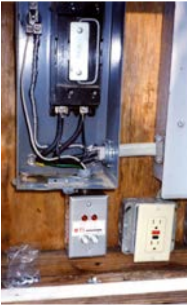
Figure 12. A surge protector covering the electrical lines in a house, barn, or other such structure is relatively inexpensive to have installed. With two or more electrical service boxes, each will need one. The surge protector includes one or more LED lights which indicate whether or not it is properly functioning. In areas of frequent thunderstorms, the unit may need to be replaced after a severe or repeated number of power surges in the line. Photo: Independent Lightning Protection Company.
